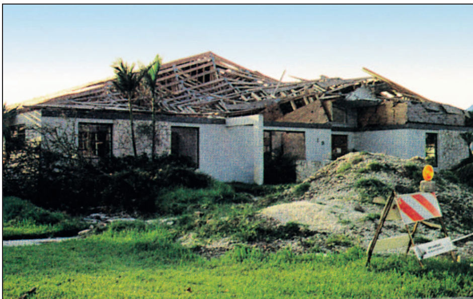
Figure 9-21. Gable-end failure, Hurricane Andrew (Dade County, FL, 1992)
