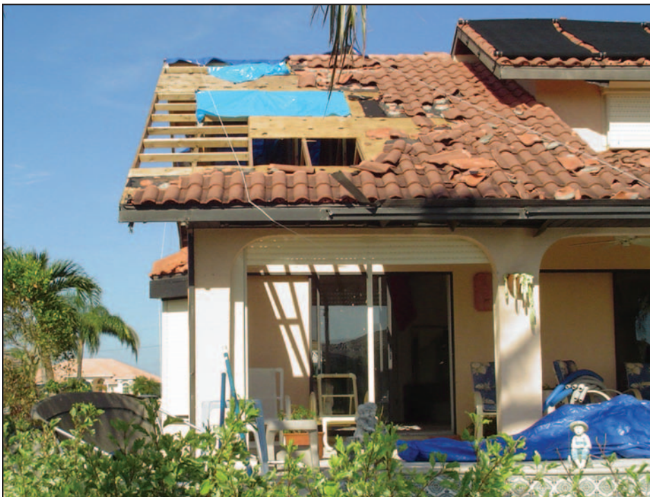
Figure 9-4. Load path failure in connections between roof decking and roof framing, Hurricane Charley (Punta Gorda, FL, 2004)
